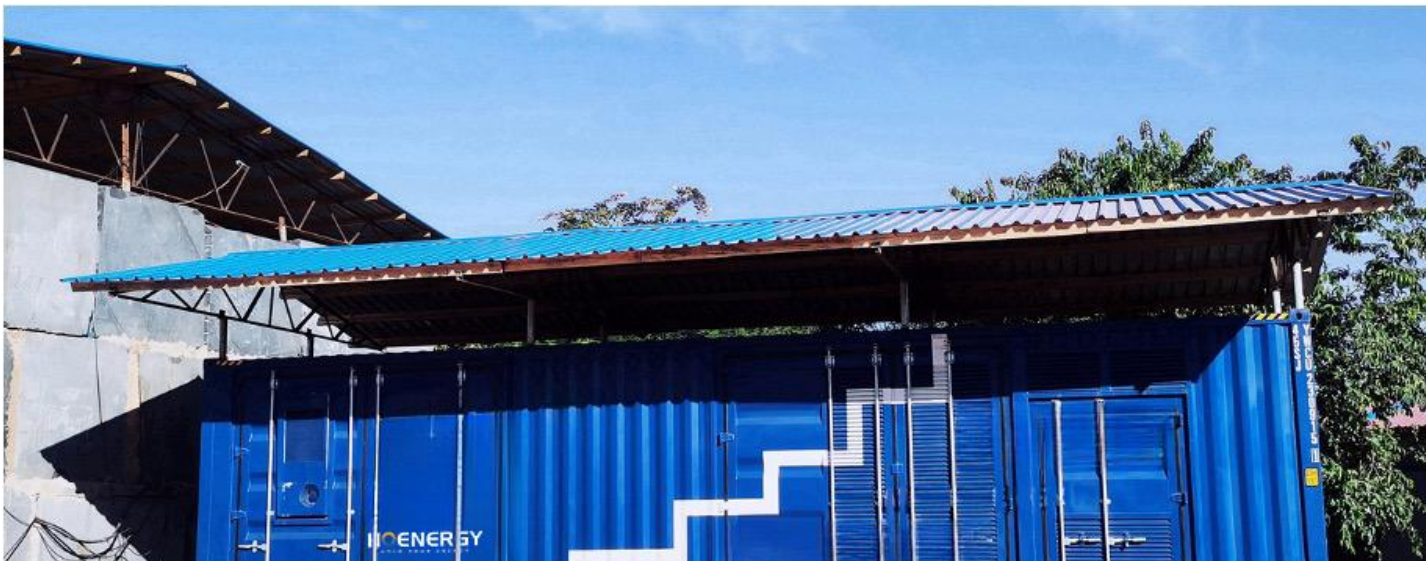
Zimbabwe Capacity--1000kW / 1290kWh
