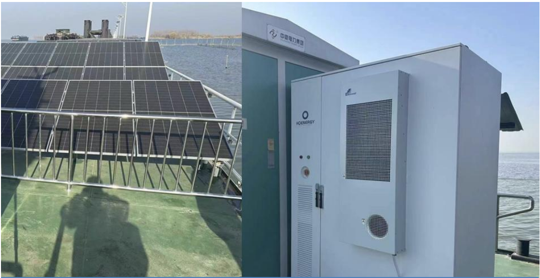
Shandong · Jining 100kW/200.7kWh
